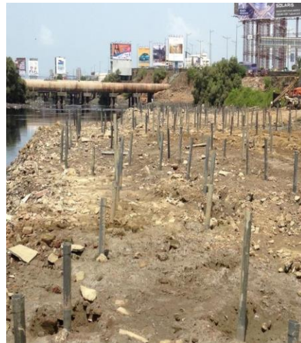
Figure 4. Holes already drilled by ODEX system in OB near water pipeline and busy road, in Mithi River Bed.
